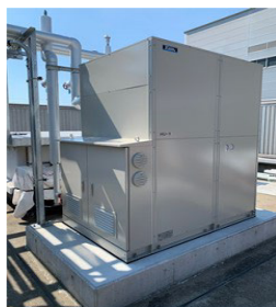
Photo. 3 Hot Water Heat Pump
