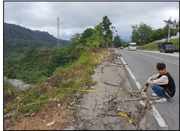
Fig. 8. Cliff Condition with road shoulder 3 meters away.
