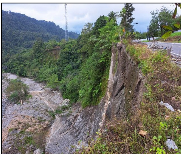
Fig. 5. Cliff condition after flash flood (may 11, 2024)
