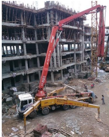
Fig. 1. Pumping concrete mixture through pipelines in the high-rise constructions in Hanoi (Vietnam)
