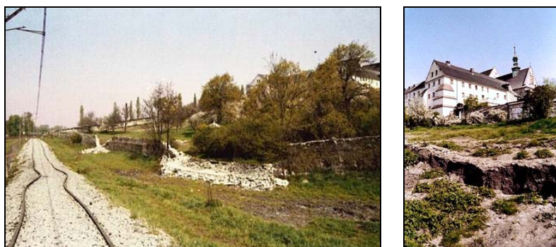
Fig. 3 Deformation of the track and destruction of the wall and cracking of the soil in the monastery's garden [4]
