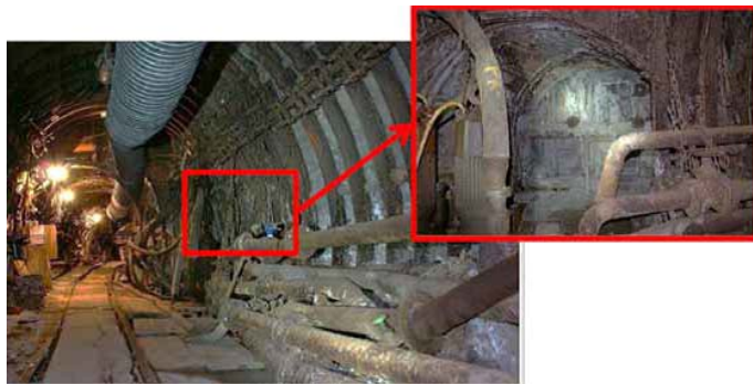
Fig. 2. Place of transverse leakage
