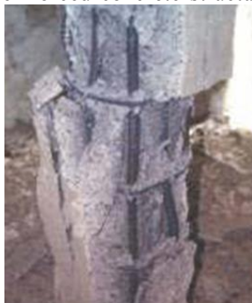
Figure 3 Reinforced Concrete Column Seriously Damaged by Fire
