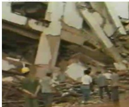
Figure 4 Totally Collapsed Reinforced Concrete Building after Fire
