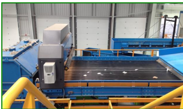
Fig. 4. Mechanical waste treatment station.
