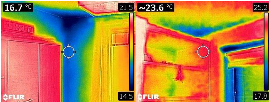
Fig. 2. Thermal image of the corner of the east gable wall south external wall and the ceiling (own elaboration).
