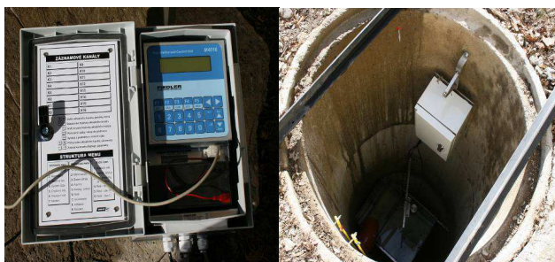
Fig. 6. M4016 Data unit in well ‘A’ [5].
