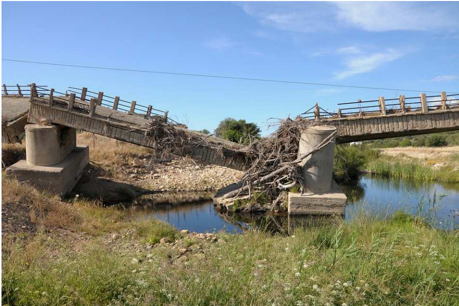
Fig. 1. Damages caused by the dynamic action of surface flood water https://pixabay.com/pl/sardynia-most-kawaler-upadek-1475156/ (access 21/02/2018)
