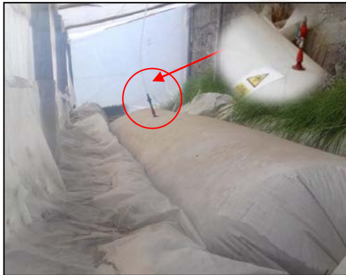
Fig. 8. Biogas output piping from the Biodigester.
