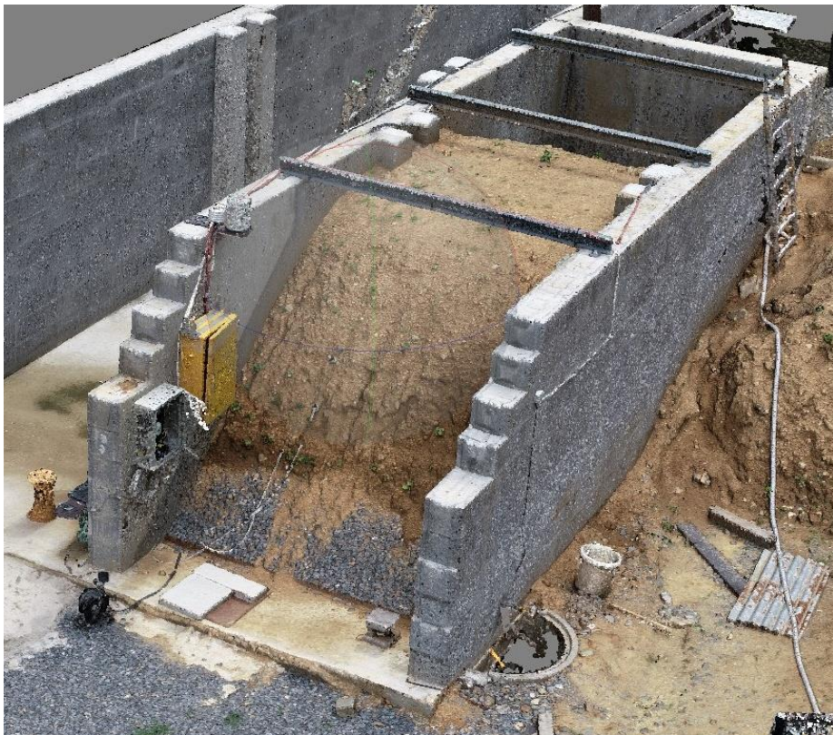
Fig. 1. View of the real-scale model of a dam as reconstructed from aerial imaging by UAS.
