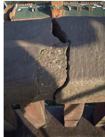
Phot. 2. Balustrade damage of the viewing platform of the Kosciuszko Mound [phot. K. Tomasziewicz].
