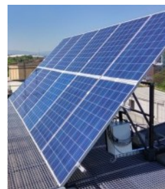
Fig. 3. Image of the PV array on the building.
