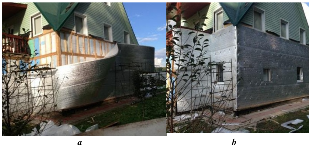
Fig. 1. The formation of the insulating shell of a frame building with the help of rolled polyethylene foam: a - deployment of a roll of IPE; b - for fixing the insulation and stitching the roll of IPE; c - formation of an isolation contour and window openings
