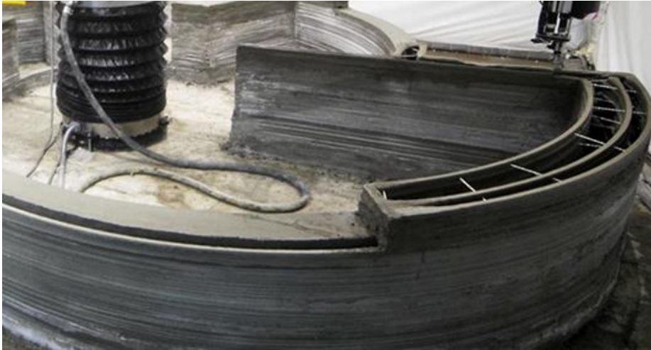
Fig. 3. General outer appearance of building walls structure made by using 3D-printing technology [5].
