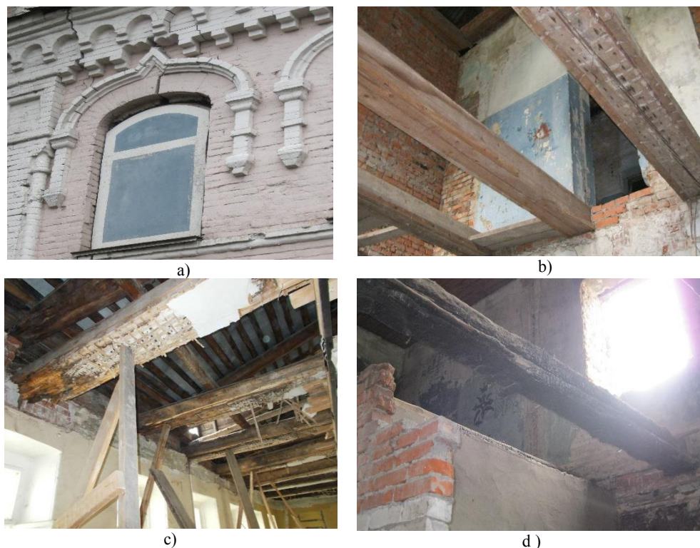
Fig. 1. Specific damages of beam structures of historic buildings:
