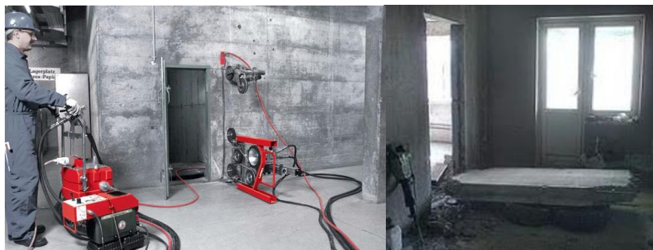
Fig. 1. Examples of unsafe increase in the width of opening in a stone wall with a wire diamond saw without its preliminary unloading and reinforcement.
