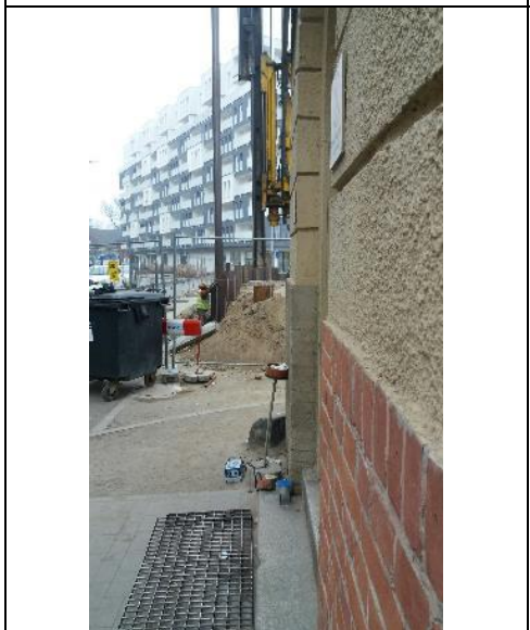
Fig. 6. Location of the sensor, plunging steel sheet piles, Dmowskiego St. in Wrocław.
