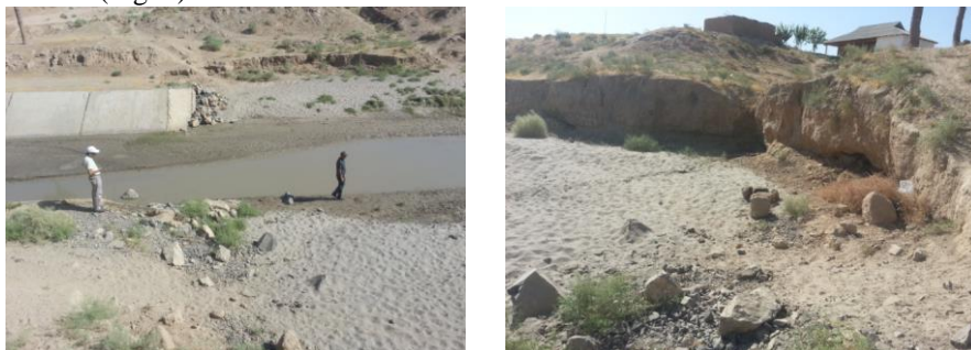
Fig. 1. Deformation processes behind the concrete part of the supply channel
