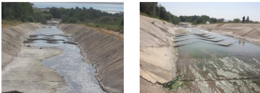
Fig. 2. Deformations in the zone of fastening of the mouth of the supply of channel
