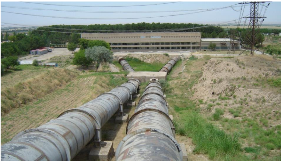
Fig. 2. Pressure pipeline of the Babatag pumping station.
