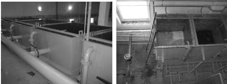
Fig. 4. Industrial filters FPZ-1 (Moscow).
