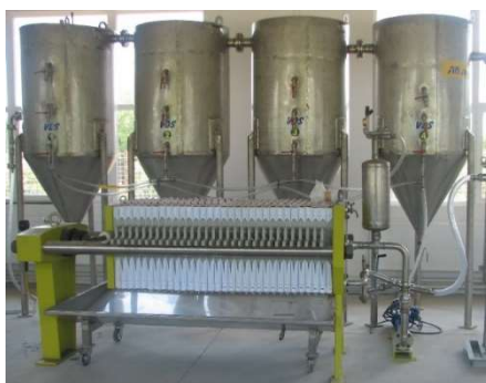
Fig. 5. Oil purification module
