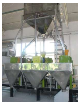
Fig. 4. Oil extraction module
