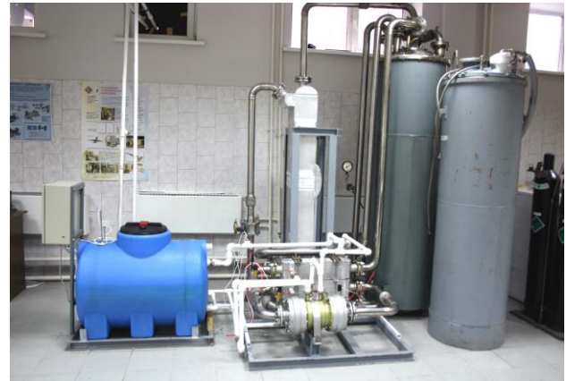
Fig. 6. General view of cryogenics cooling system.
