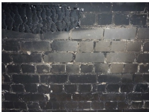
Figure 1. General view of the wall of the building after the fire.
