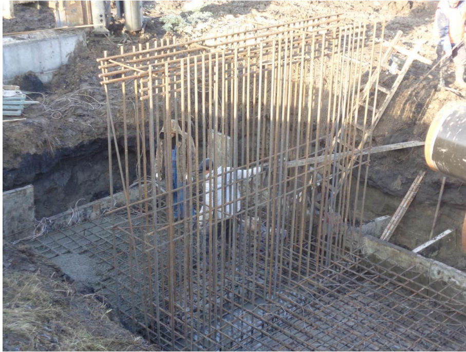
Fig. 2. All the rebar is laid out which means that this entire anchor is ready to be covered in concrete.
