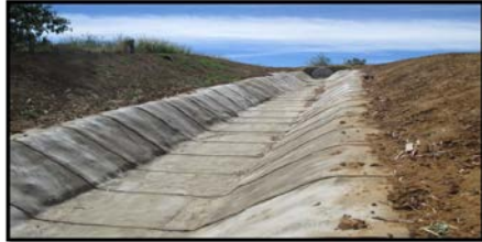
Fig. 2.1. – Concrete canvas-lined irrigation canal.
