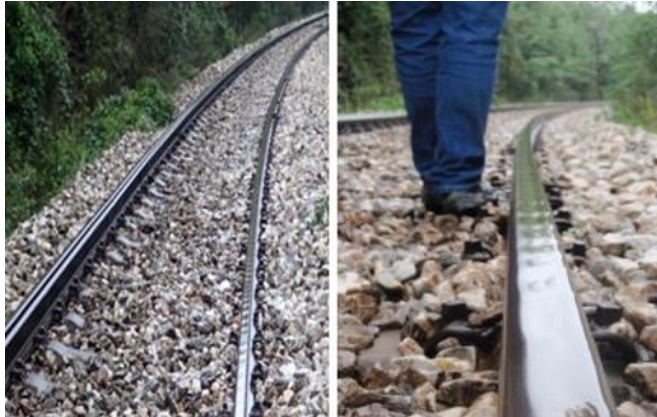
Fig. 1. Long-pitch corrugation in curve with radius R = 300 m (railway section Resnik - Bela Reka for mixed traffic).
