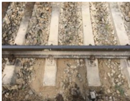
Fig. 4. Mechanism of superstructure deterioration (Pančevo Varoš station, May 2017).
