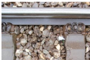
Fig. 6. Sleeper damage during track tamping (railway section Resnik - Bela Reka).
