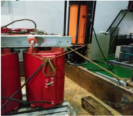
Fig. 3. Field test layout of dry transformer winding.
