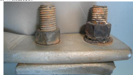
Fig. 10. Morphology of the failed clamp bolt.
