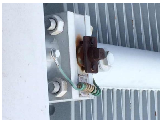
Fig. 4. Corrosion morphology of butterfly valve bolts.
