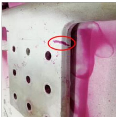
Fig. 3. Crack penetrates to the side
