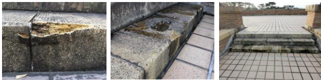
Fig. 1. Lump exfoliation of Nikkaseki at rooftop steps. (2018)
