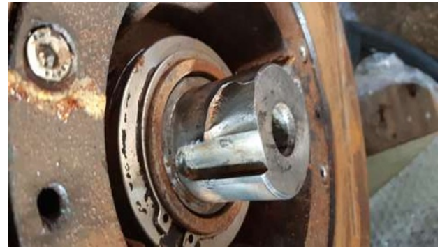
Fig. 2. Electric motor shaft damages by pump impeller.
