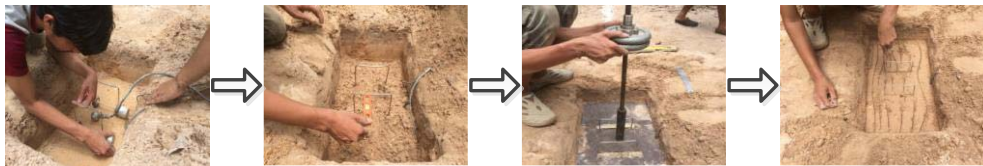
Fig. 4. Field device installation and configuration.
