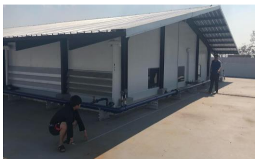
Fig. 2. Roof of the female dormitory used in simulation and the orientation of PV panels.
