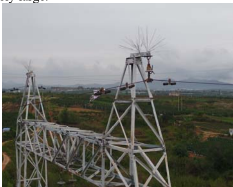
Fig.1. Bird repellent belt on overhead ground wire
