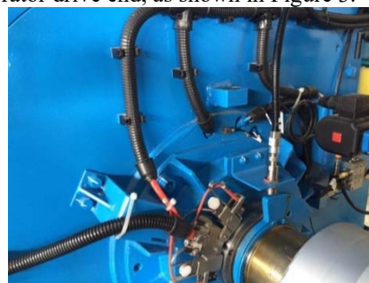
Fig.3 The Acceleration Sensor Is Installed At The Drive End Of Generator
