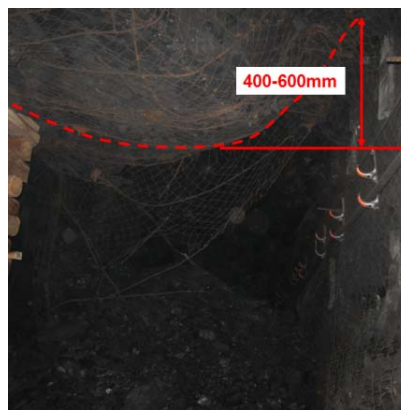
Fig. 2 Severe roof deformation and failure during secondary mining
