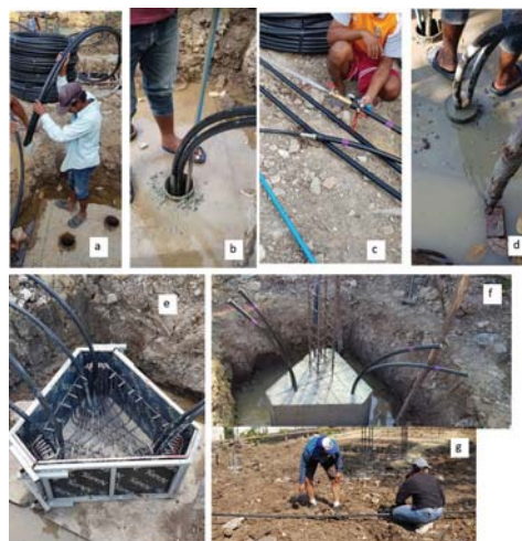
Fig. 11. Installation of HDPE U-tube loops in the steel pipe piles of a residential house in Bangkok
