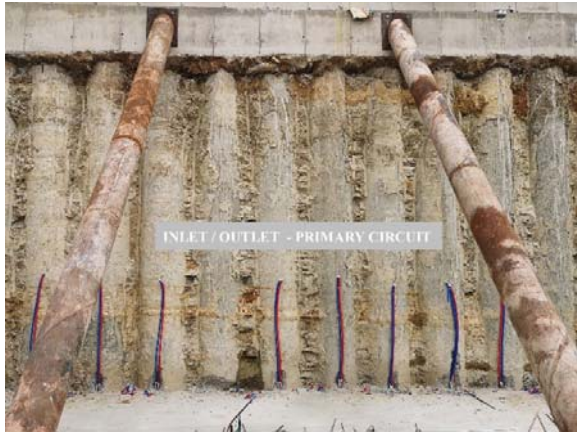
Fig. 7 Inlet and outlet of primary circuit at the bottom of excavation level at the extraction stage
