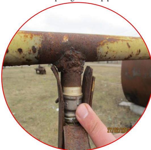
Fig.4. Unauthorized tampering into the gas distribution pipeline.
