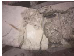
Fig. 3 crushing of concrete
