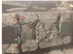
Fig. 5 carbon plate is broken
