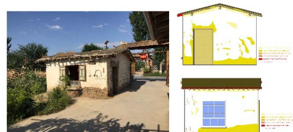
Fig7. Investigation and analysis of Building 2 disease
