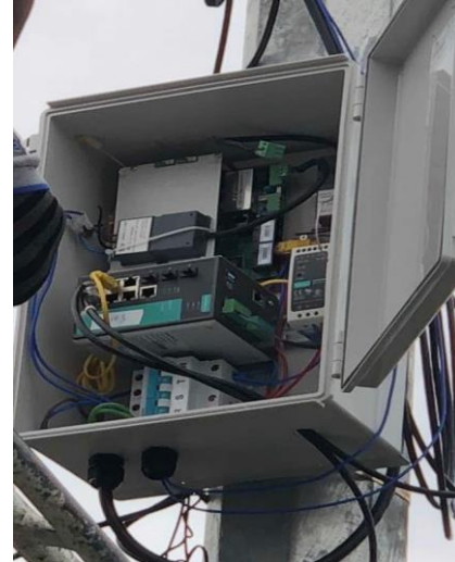
Fig. 3. Head End (HE) on the electrical pole.
