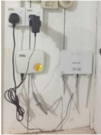
Fig. 5. CPE installed with wireless modem at Rumah Jimbun.
