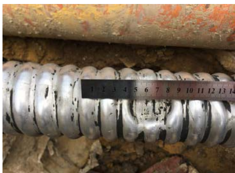
Fig. 3. Damaged aluminum sheath
