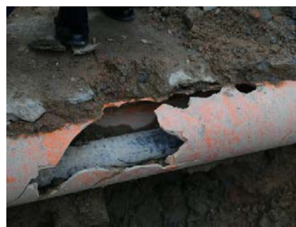
Fig. 1. buried tube after mechanical damage.
