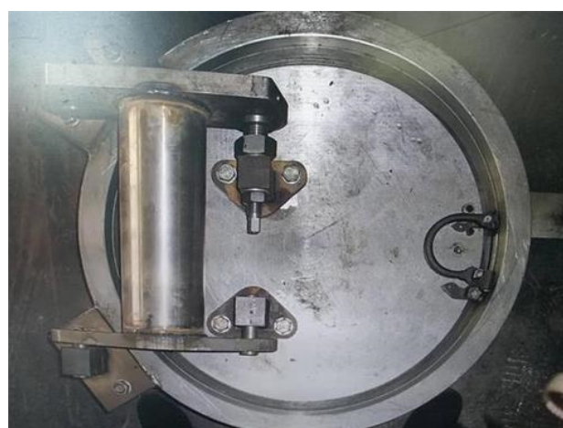
Figure 5. Safety Interlock Unit
