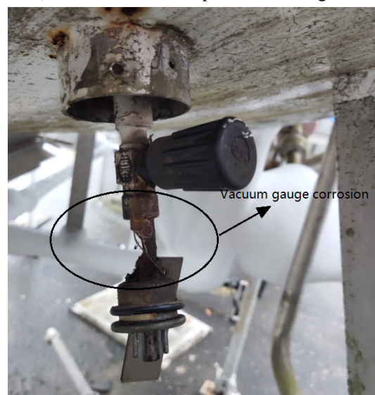
Figure 2. Vacuum gauge corrosion
