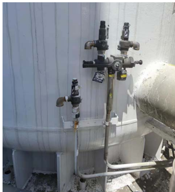
Figure 4. Safety valve and Rupture Disc of LPG Storage Tanks
