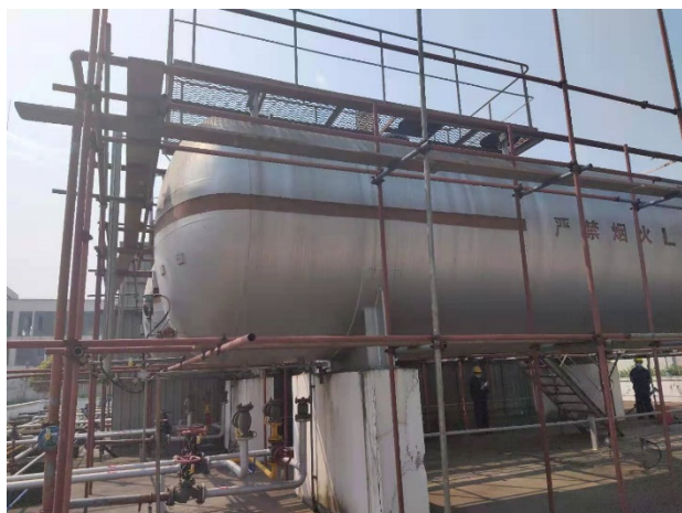
Figure 3. LPG Storage Tanks
