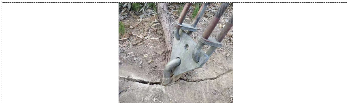
Figure 6. Cracks occur on the ground near the ground anchor on the right side of the small-number-side of #94 tower, and the degree between ground anchor and ground is larger than that of cable and ground.
