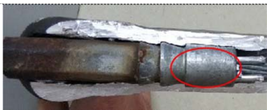
Figure 3. There is no rust on the surface of the steel anchor inside the aluminum casing.
