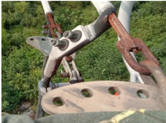
Figure 6. Comparison of corrosion of tensile steel anchor with other metal fittings.
