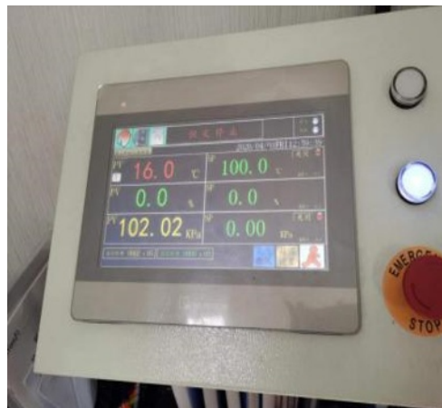
Fig. 5 Temperature and humidity display panel of the normal temperature comprehensive test system in container laboratory
