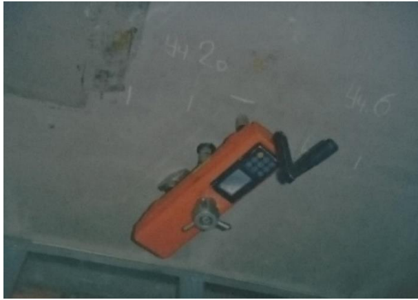
Fig. 2. Performing slab test from a bottom out by the separation with spalling method using the “ONIKS-OS” device
