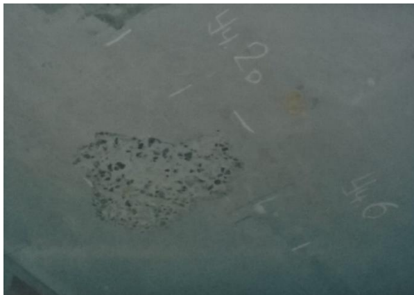
Fig. 3. View of the area after the separation with spalling test.
