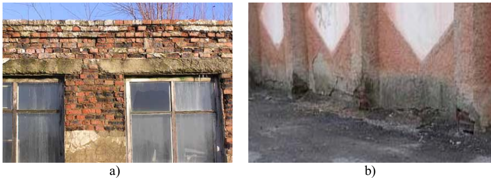
Fig. 4. a) thawed and destroyed to a considerable depth sections of external brick walls; b) destroyed pilasters in the wall of the gym in those places where the blind area is adjacent.
