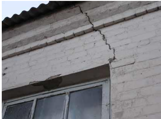
Fig. 5. Cracks above the aperture in block 1.
