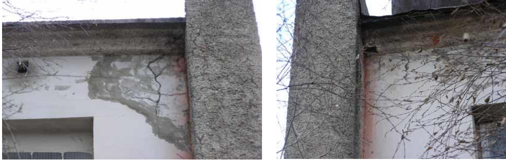
Fig. 3. Through cracks 2-3 mm wide in block 3 of the school complex.
